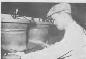
Henry N. Nichols, welding foreman is considered an artist with a torch.
